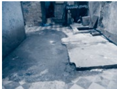
Above and right: leaking sewage fills corridors and causes a health hazard for residents.
